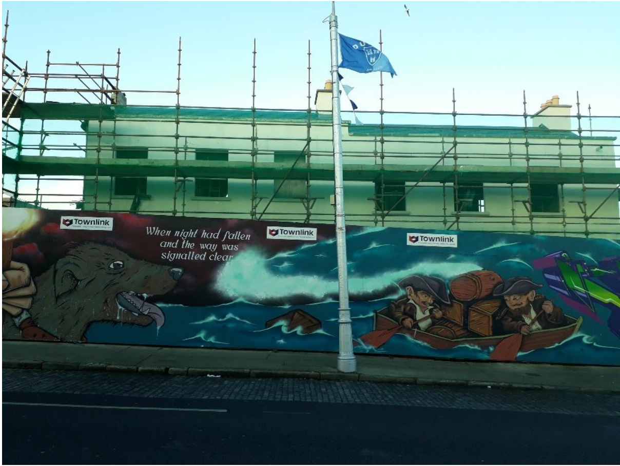
Works on the frontal rendering and brickwork to the front of 1-6 Ballybough Road continues and is due for completion by February 2019.
